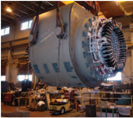
Generator wound stator ready for VPI.
