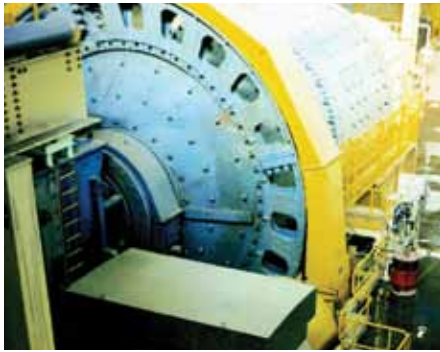
Synchronous motor driving a ball mill.
