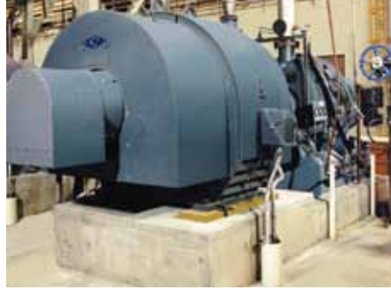
Synchronous motor with PMDP™ enclosure driving a refiner.
