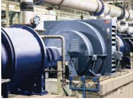
Vacuum pump drive
