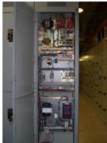
Regutron III Installed in Existing Panel
