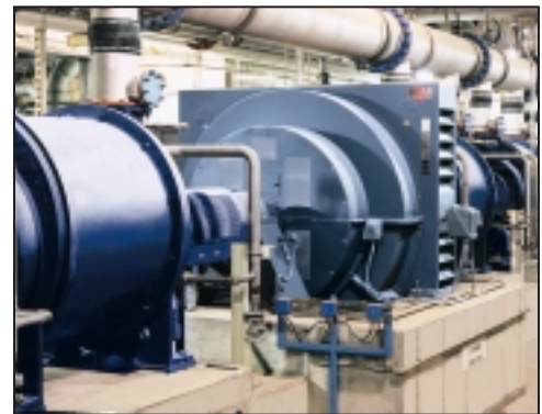
Vacuum pump drive
